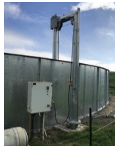
Submersible Stirrer and Over the Wall Stirrer Frame on Tasman Tank.
