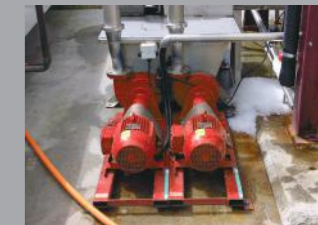
Horizontal Pumps at Chicken processing facility
