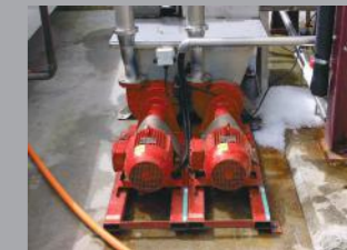
Horizontal Pumps at Chicken processing facility
